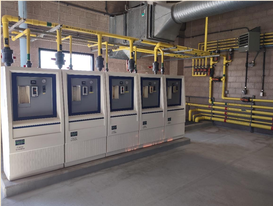
Replace Chlorine Room Chlorinators
