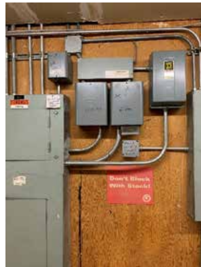
Existing lighting control time clocks and contactors
