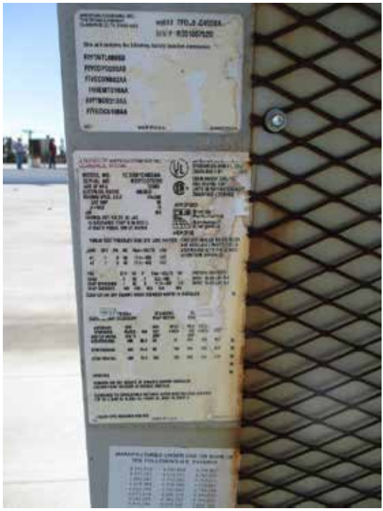
Existing Rooftop Unit Nameplate
