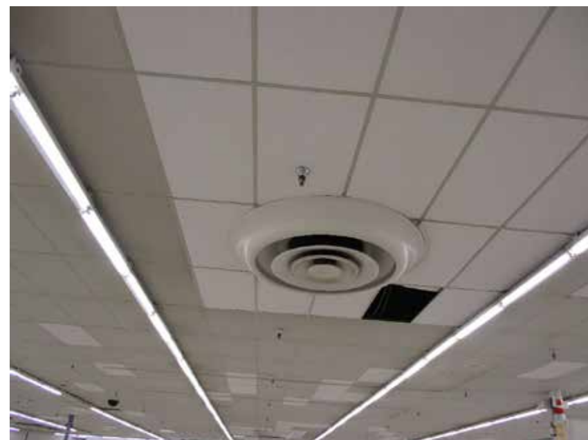
Existing Supply Air Diffuser
