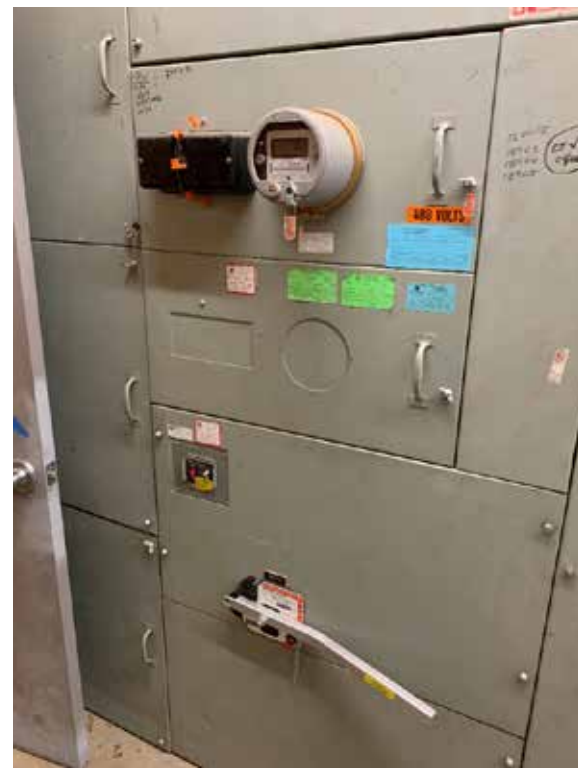
Existing Service Entrance Section
