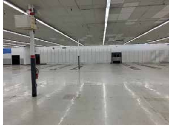
Existing fluorescent strip lighting
