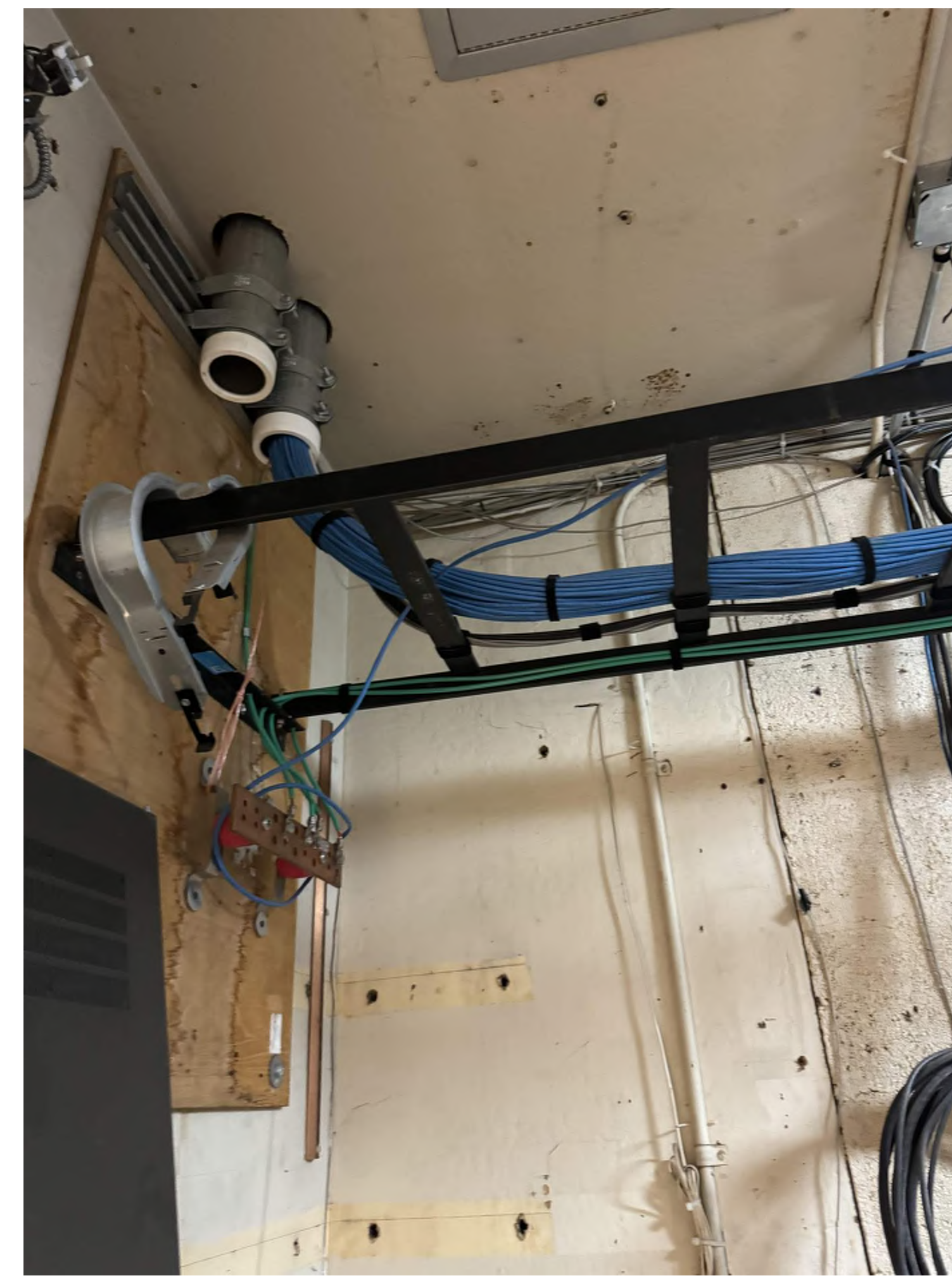
03 VIEW OF IDF ROOM - SOUTH WEST CORNER
