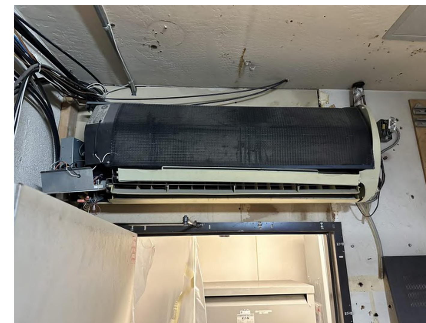
07 VIEW OF AC UNIT ABOVE DOOR (SOUTH)
