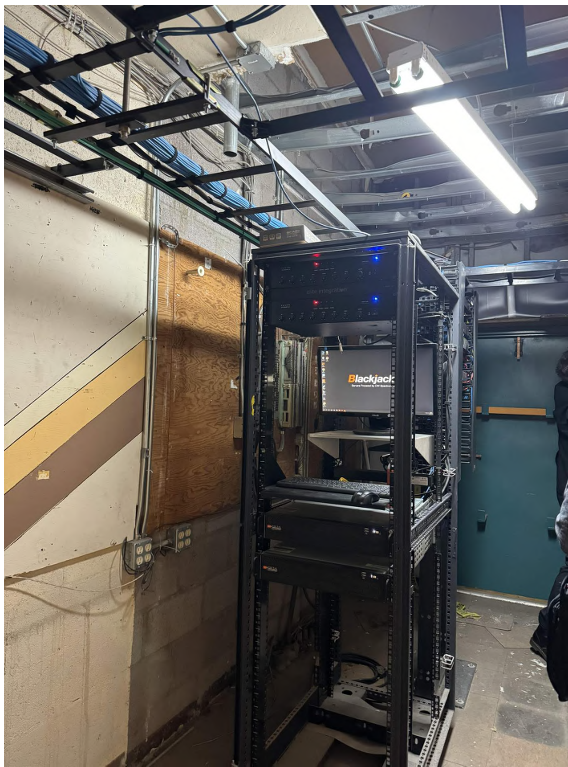
01 VIEW OF IDF ROOM (LOOKING NORTH WEST)
