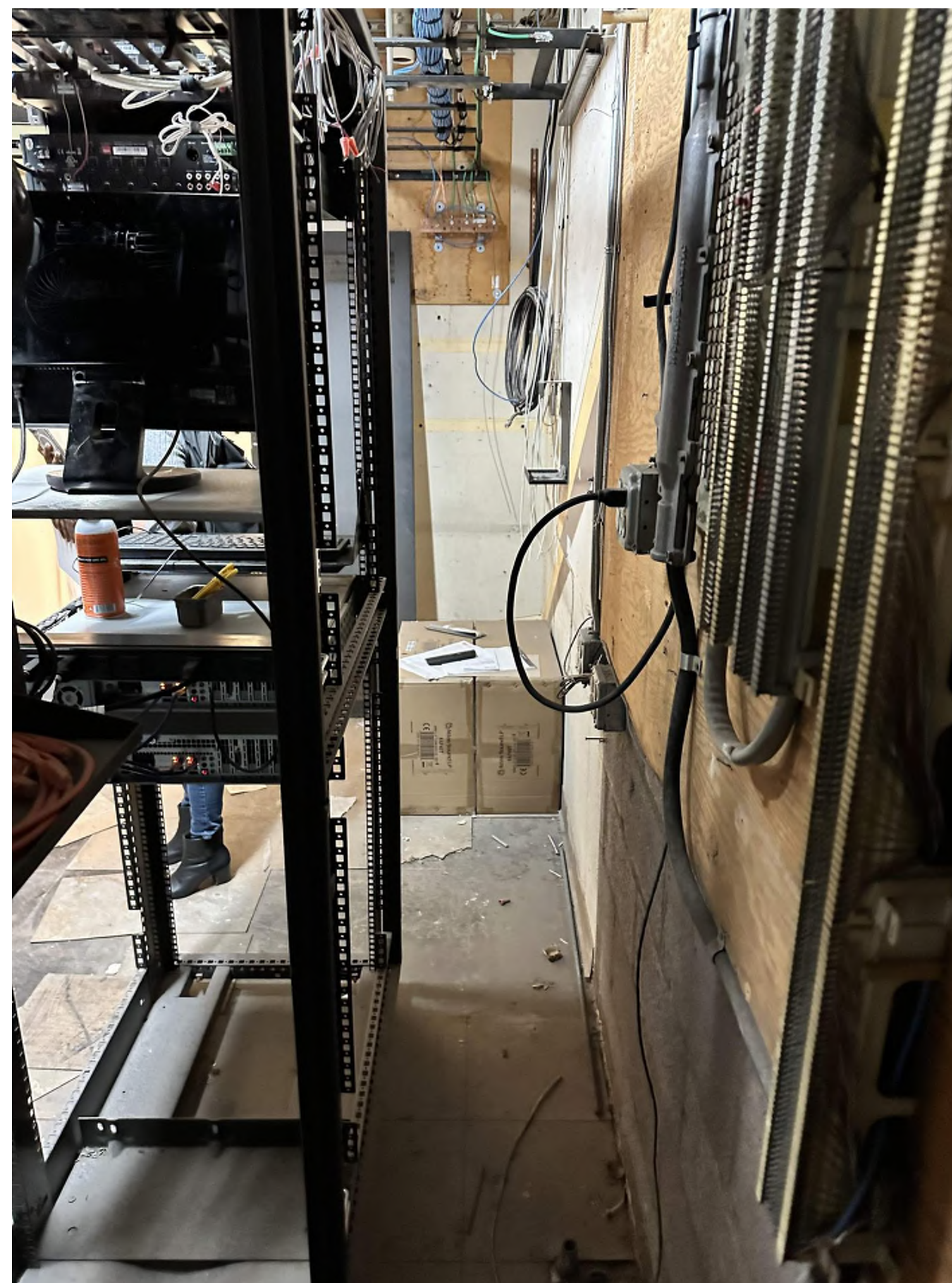
02 VIEW OF METAL SHELF FOR SERVER UNITS (LOOKING SOUTH EAST)
